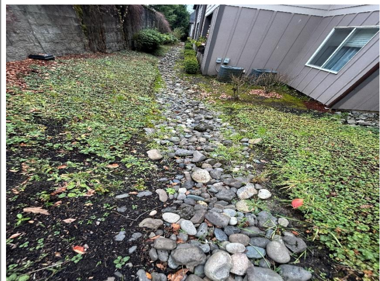
8.8 Detail of the French Drain system at the back of the East elevation of the property.
