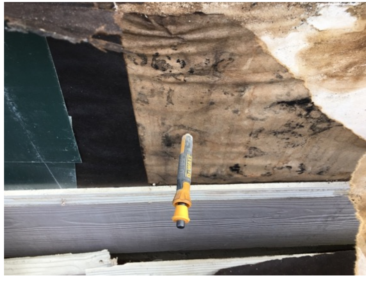
1.10.14 Demonstration of deteriorated gypsum sheathing.
