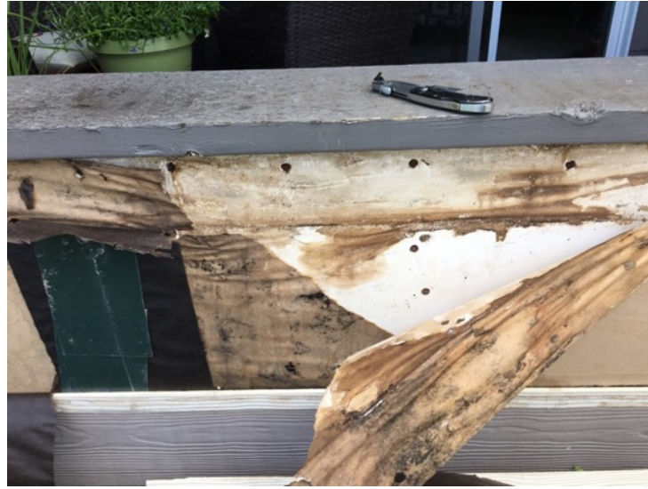
1.10.13 Deteriorated gypsum sheathing.
